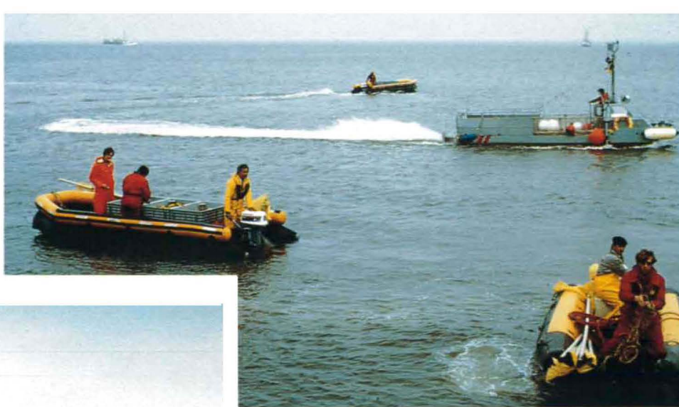
Bay cable operation
